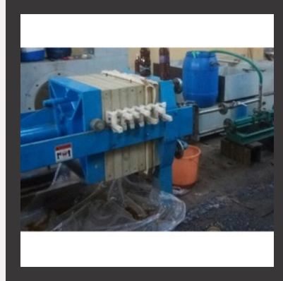
Filter Feed Pumps
